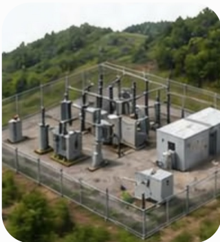
6 Switchyard and auxiliary facilities
