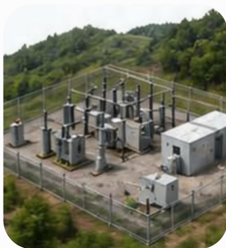
6 Switchyard and auxiliary facilities
